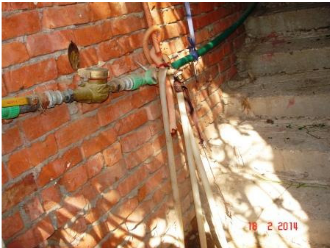
Another water meter to the first and second floor
