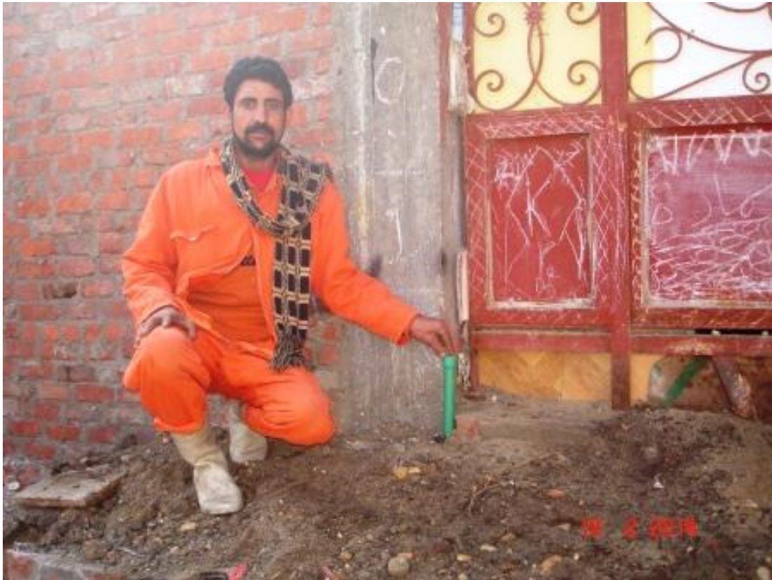
A new attached pvc tube to another home
