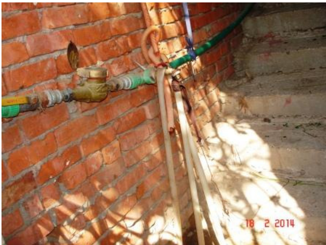
Another water meter to the first and second flour
