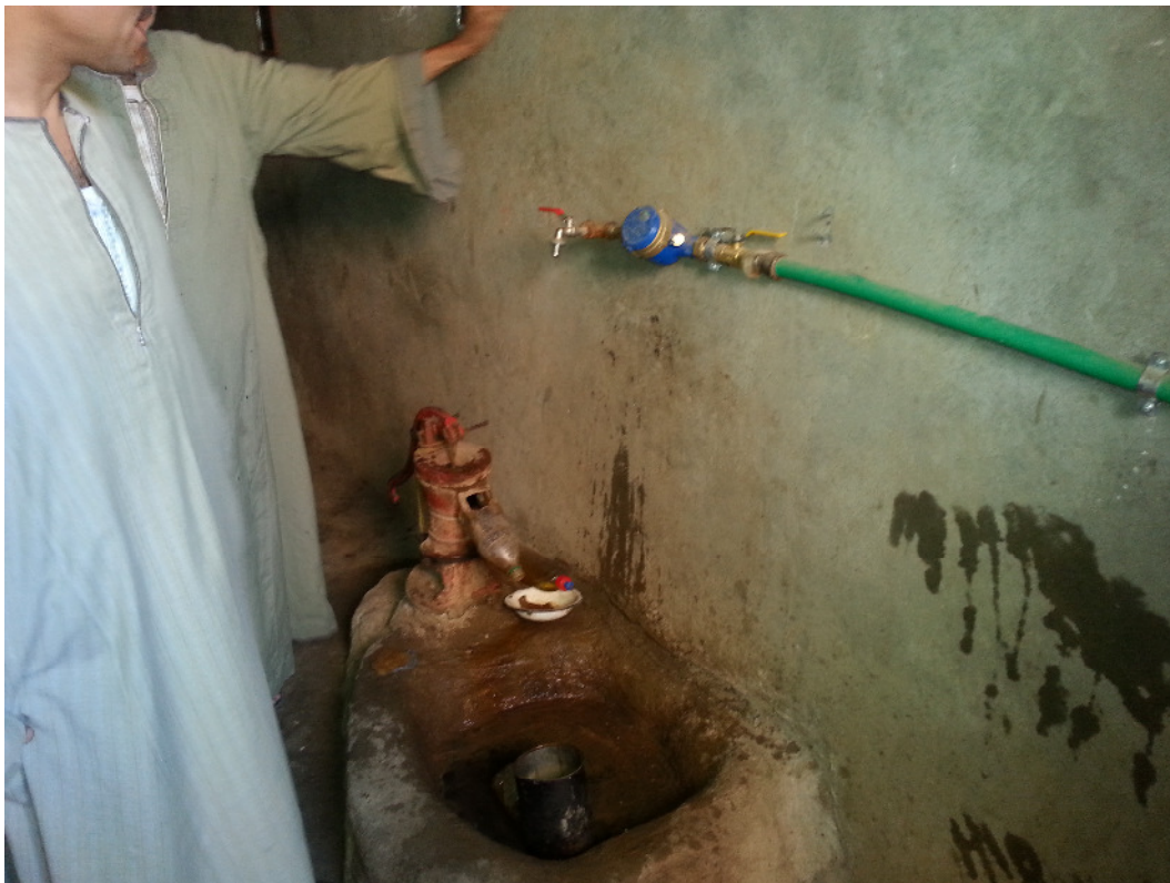
New drinking water connection with water meter
