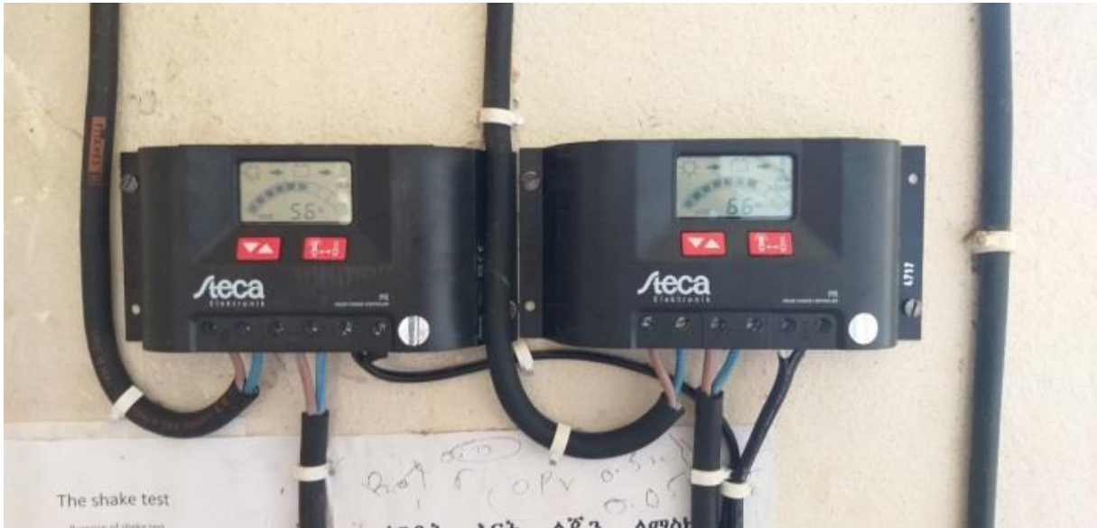
Charge Controller for fridge batteries
